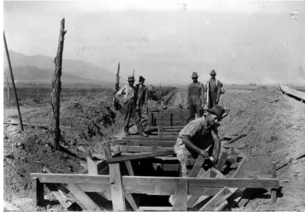
Photograph 13. Construction work on a Highline Canal lateral located north of Santaquin Circa 1915.
